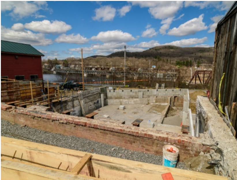
Construction site at Bellows Falls Garage. Photo courtesy of Windham & Windsor Housing Trust/Liz LaVorgna
