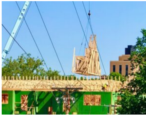
Crane lifts building material to an apartment complex in midtown Omaha. (Cindy Gonzalez/Nebraska Examiner)
