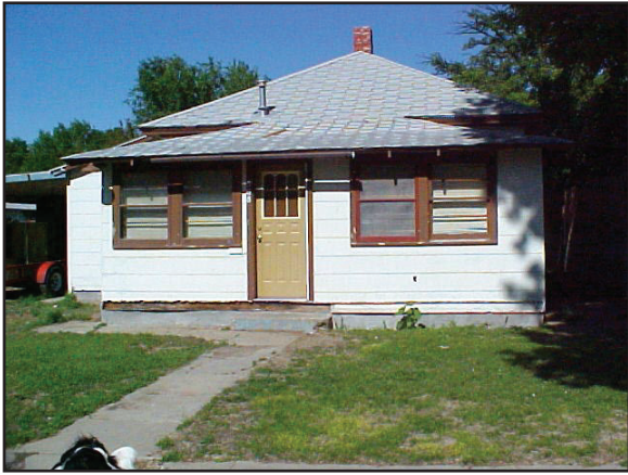
Before & After of an exterior rehabilitation in Basin, WY including a new roof, exterior doors, paint, sidewalk, and a new lawn.
