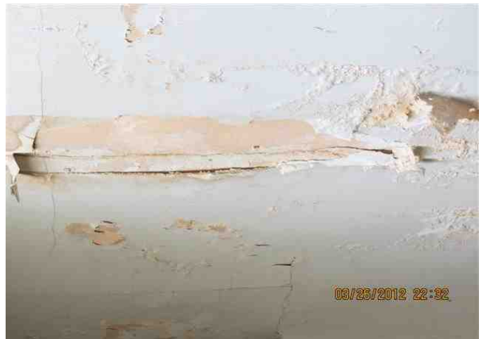
16872113_60.JPG: Ceiling damages. Interior is
