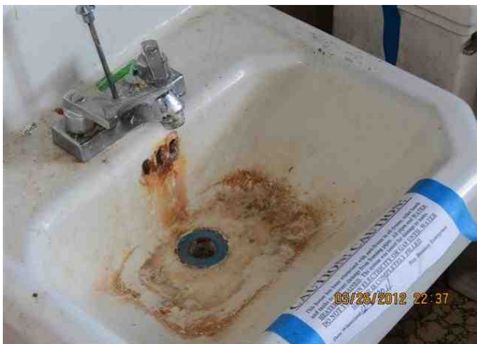
Interior #11 16872113_85.JPG: Sink - unsure why there is so much
