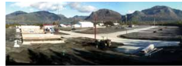
The Raven Loop Extension Project in Metlakatla, currently in Phase I, is primarily infrastructure development for 16 low-income rental apartments, two fourplexes, four duplexes and 13 single-family homes.
