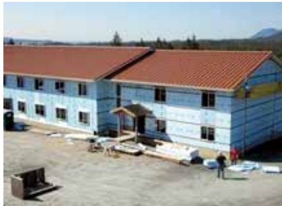
Construction on the new 17-unit, low-income Saxman Senior Center began in May 2010. The project is a partnership with the Tlingit Haida Regional Housing Authority (THRHA), the Organized Village of Saxman, and the City of Saxman. Funding for the $6.7 million project included ARRA funds awarded to THRHA and the village of Saxman, HUD Indian Housing Block Grants, and AHFC supplemental housing funds. Estimated project completion is early 2012.
